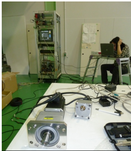
The control system fabricated by Kobayashi
