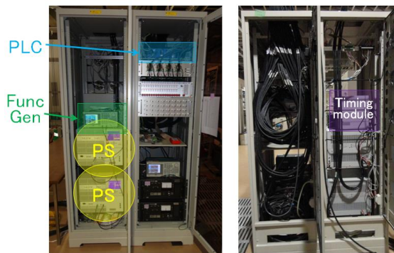
Figure 2: Control rack of skew quadrupole magnet.
