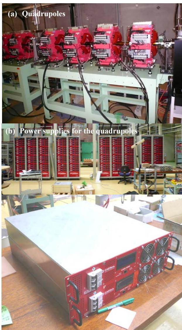
Figure 4: Quadrupoles and power supplies.
