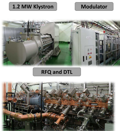
Figure 2: RF source and accelerating structures.
