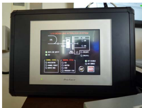
Figure 6: Main controller for LCS.
