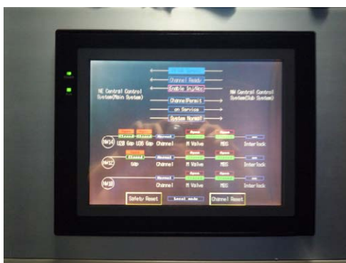
Figure 4: Central control system for PF-AR.
