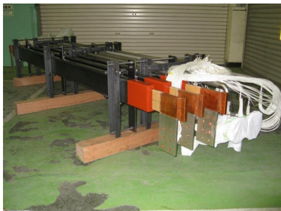
Figure 9: P6 utility duct (signal cable ducts, electric power bus ducts, water pipes, a vacuum pipe).
