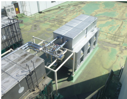
Figure 1: New cooling tower.
