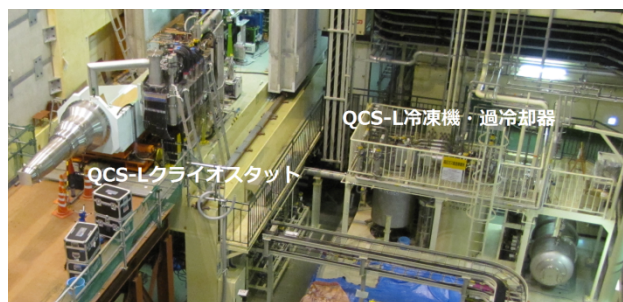
Figure 12: QCS-L cryostat and He refrigerator.
