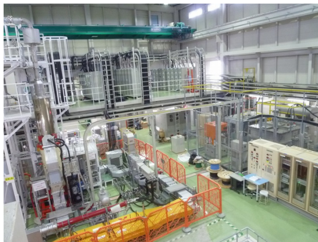
Figure 2: High-power rf system in the building for positron damping ring (PDR).
