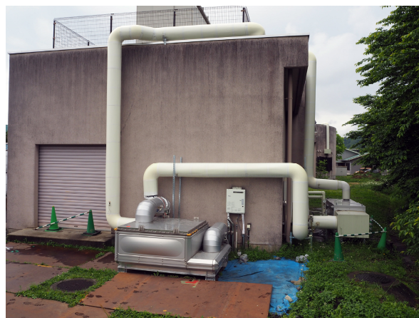
Figure 7: A utilization site of thermal storage tank at Kanuma welfare center "Deainomori".
