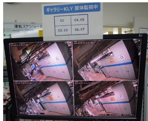
Figure 2: Surveillance video of klystron power supply.
