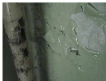
Figure 2: Peeled epoxy coating at \mu -monitor.
