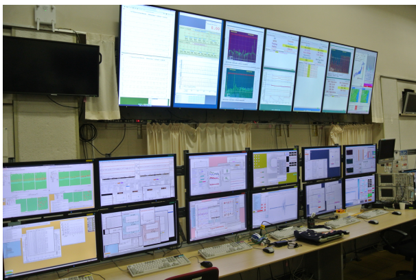
Figure 4: Consoles and monitors at SuperKEKB control room.
