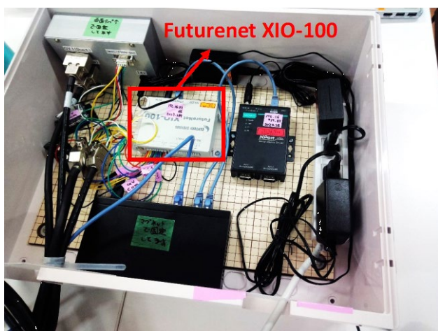
Figure 4: A signal interface box with an XIO-100 module.
