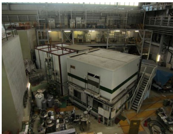
Figure 3: Air conditioner installed in the North Counter Hall.
