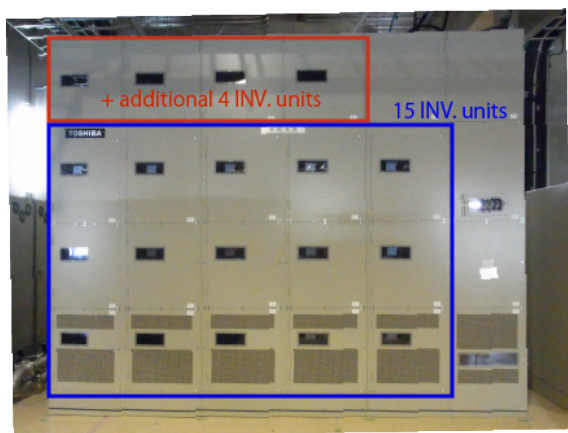
Figure 1: Anode power supply with 19 inverter units.
