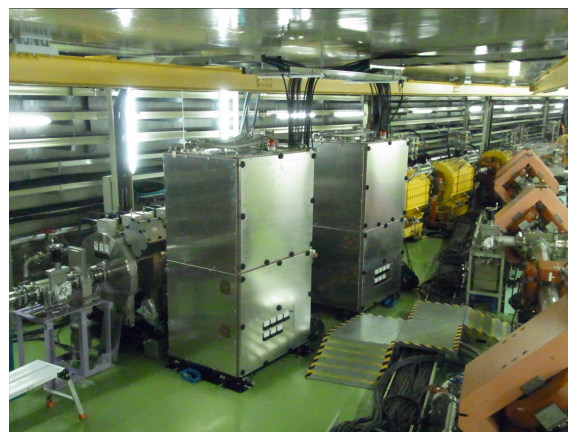
Figure 2: Two 2 nd harmonic RF cavities with FT3M.
