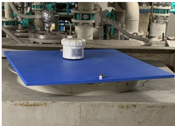
Figure 1: Ultrasonic level gauge on the buffer tank of cooling water system.
