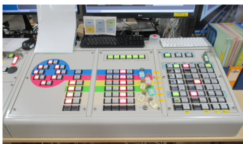
Figure 12: Consol of the safety system.
