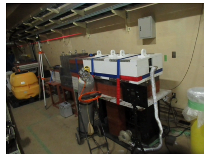
Figure 6: The beam dump at the end of injector linac.
